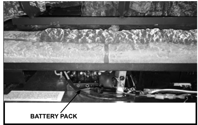
Figure 6.3 Battery Pack Installed
